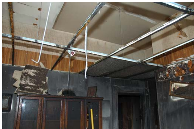
Work done under the Retro-fit section of the Fire Code contained the fire to this unit and prevented fire spread to the remainder of this 3 storey building.
